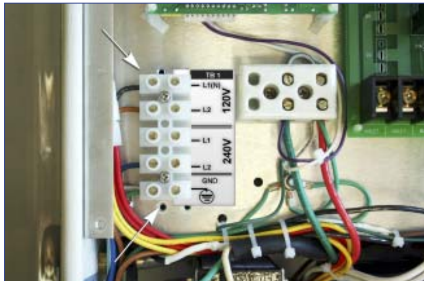
Figure - 10 Terminal Block
